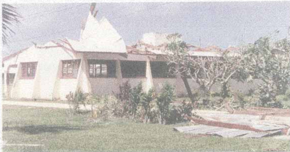
TOP - Beulah College classroom block with roof uplifted.
