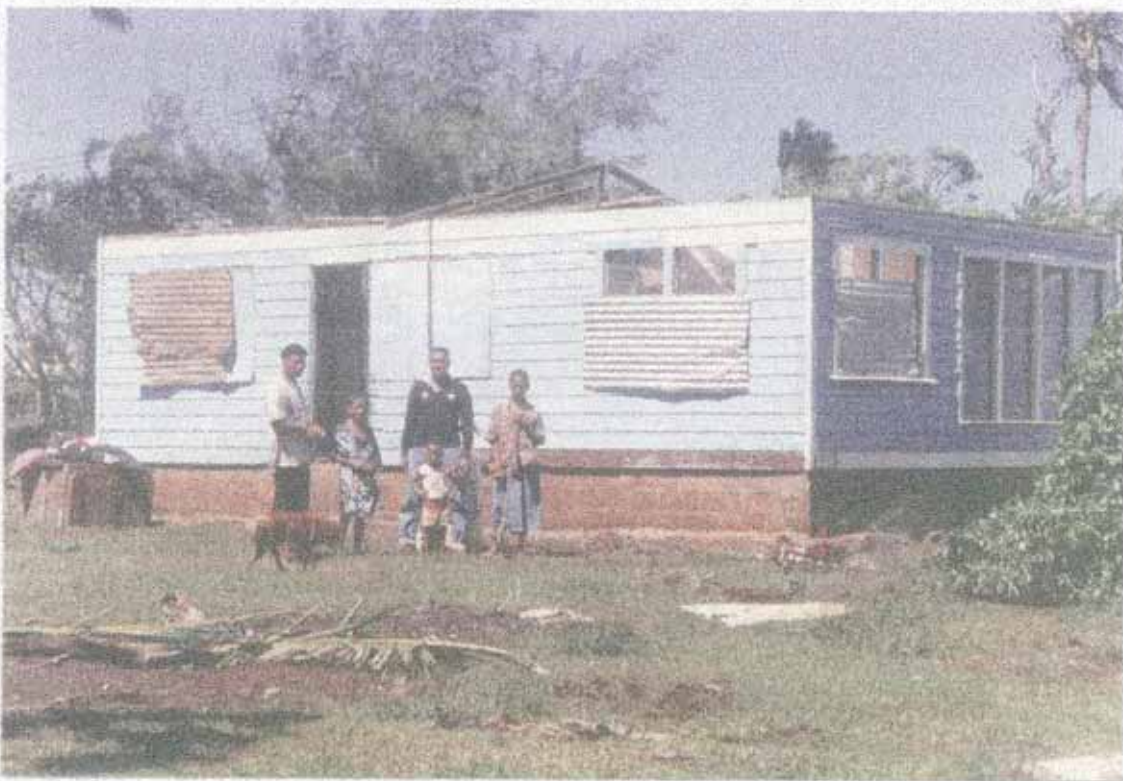
BOTTOM - Tropical residential roof damages due to absence of cyclonic ties.
