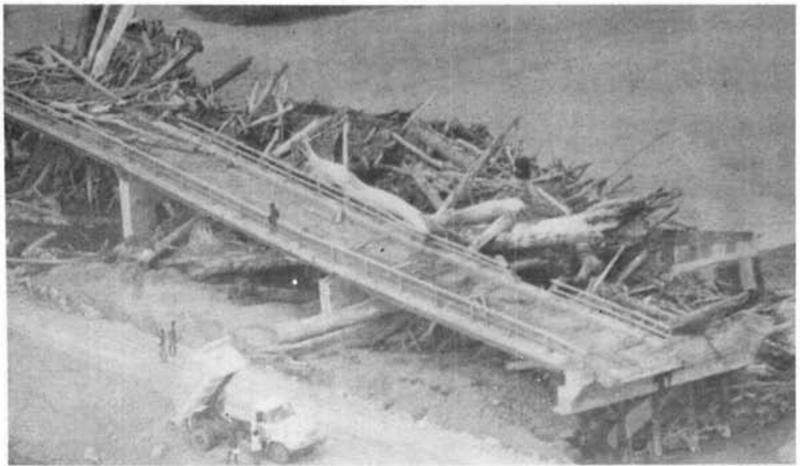
FIGURE 6. HUGE LOGS JAMMED AGAINST THE DEVASTATED NGALIMBIU BRIDGE, GUADALCANAL.
