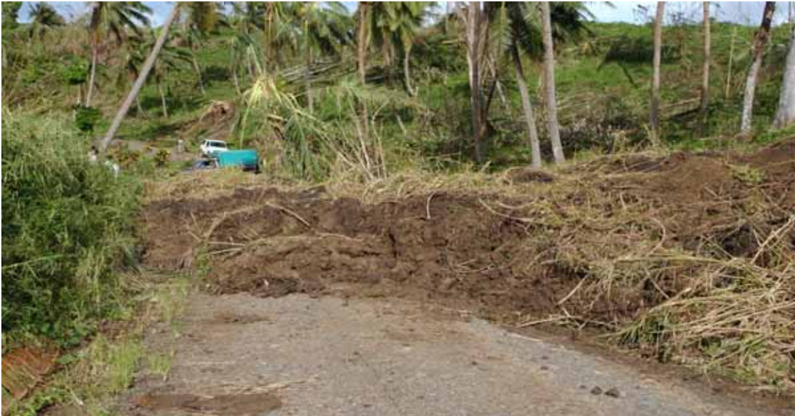
Inaccessible road caused by landslide/debris blockage
