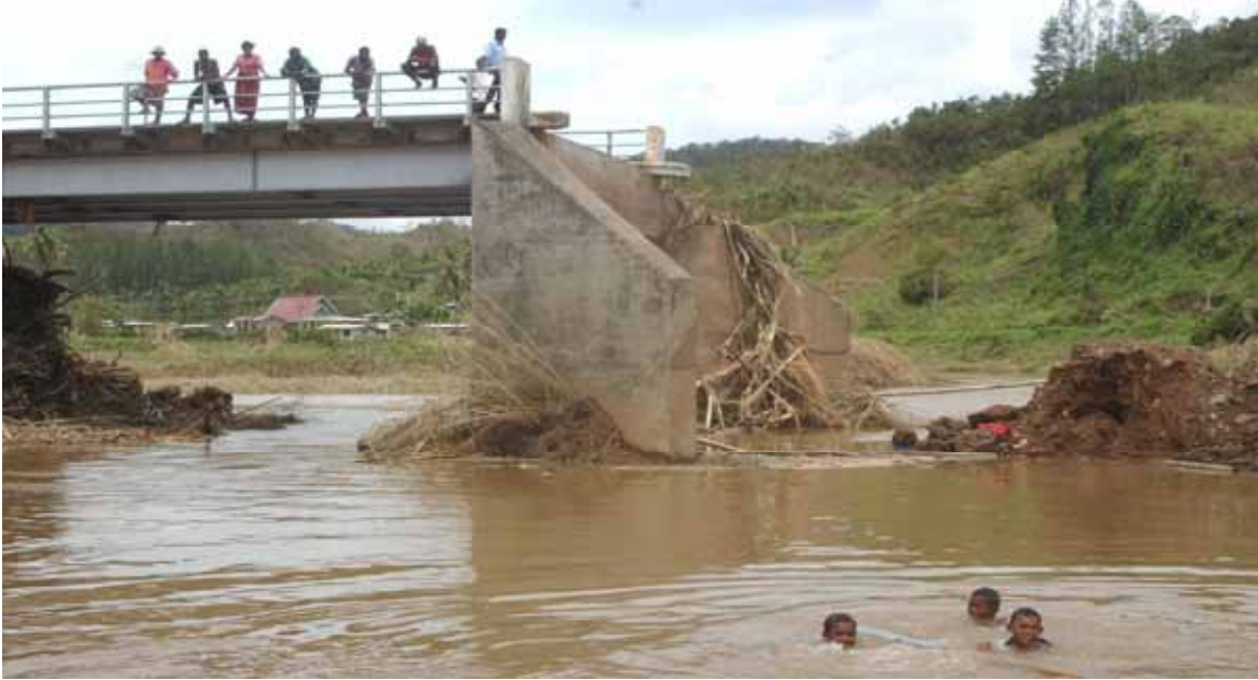
Broken Vunivesi bridge in Savusavu
